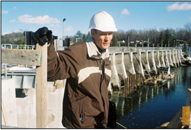
Photo: Robert Fleming International Research Inc. / John Wynsma, Project Engineer, Innergex, inspects the new 8.0 MW Glen Miller power station being completed at Trenton by Innergex of Longueuil, Quebec
